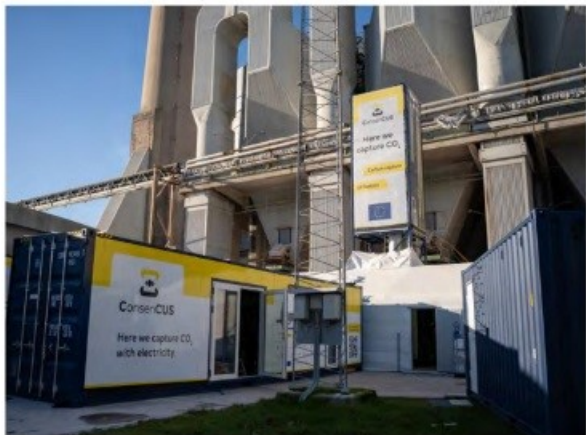
Pilot CCS unit installation underway at Aalborg Portland (Cemantir Subsidiary), with ongoing feasibility studies at selected plants.
